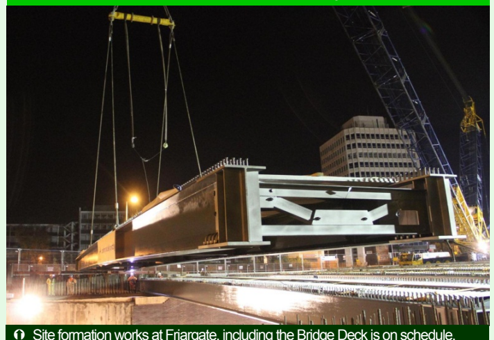
Site formation works at Friargate, including the Bridge Deck is on schedule.
